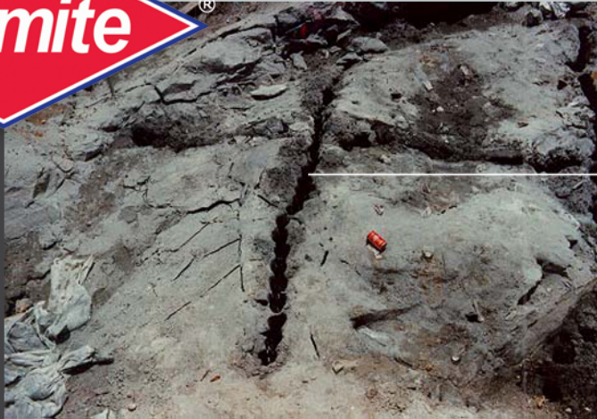
Continuous slots cut into the rock to create a free break face.
