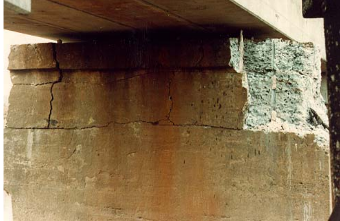
Cracking to cold joint and depth of drilled holes
