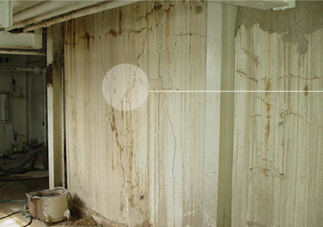
• Cracking in foundation as seen from basement.
